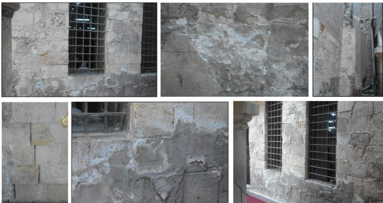
Fig. 3: Mortar damage patterns in the El-Ashmaoi Mosque
